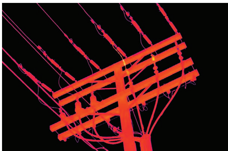
Electrical utility distribution lines
