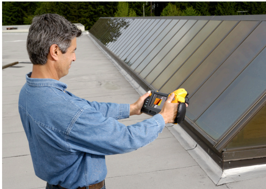
Facilities manager checks the roof flashing to make sure there is no moisture penetration.
