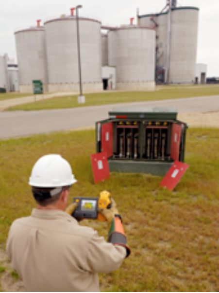
Bringing thermography in-house allows Weyh to help protect expensive equipment by scanning the ACEC-owned facilities on the sites of key co-op members.
