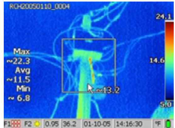
Taking a thermal image of this pole top located on a dairy farm made it easy to see that there was a problem.
