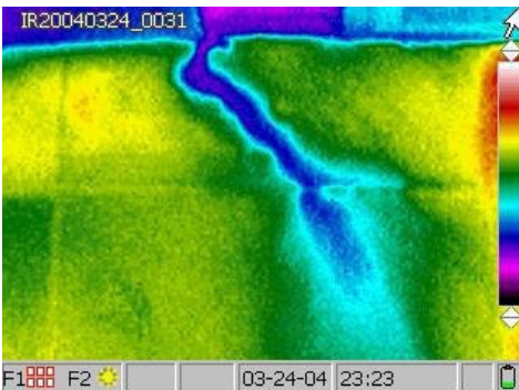
Water running underneath the tile deck into the unit below.
